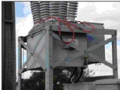
Figure 5 – Installation of neutral flexible TC on recloser ESV 3810 with Electronic control
