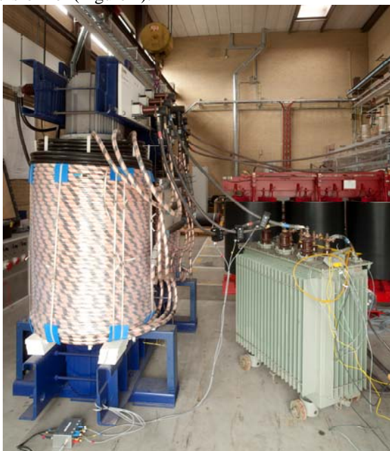
Figure 4 A 250kVA MV/LV transformer (right) in combination with a fault-current limiter (left) undergoing thermal testing under severe harmonic conditions in the FPGLab
