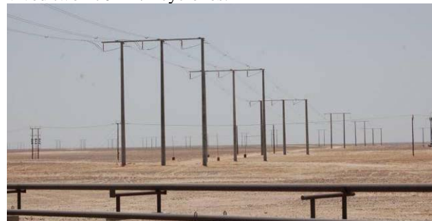
Fig. 2: HV poles in service in Oman.
