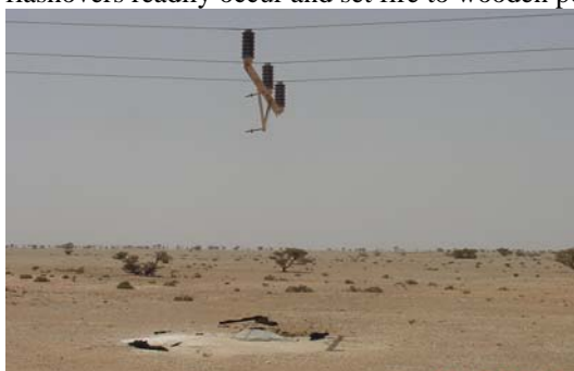
Fig. 3: Remains of a wooden pole after a fire.
