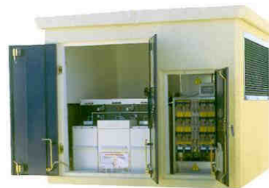
Figure2 – Example of MV/LV compact substation.
