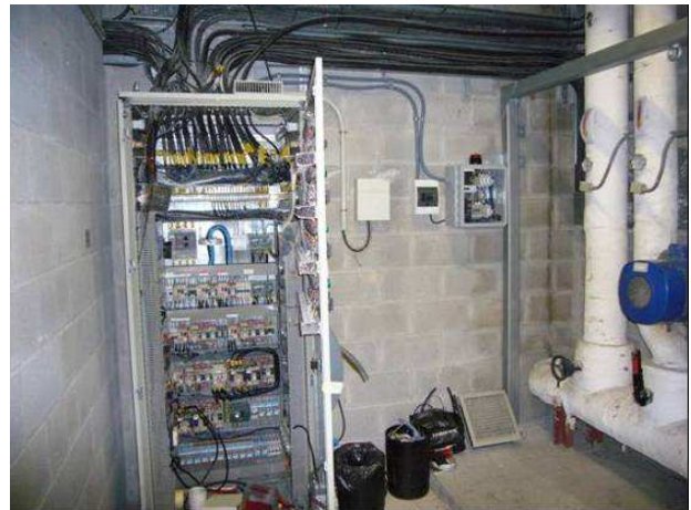
Figure 3 OPTIGES local controller installation in Bilbao
