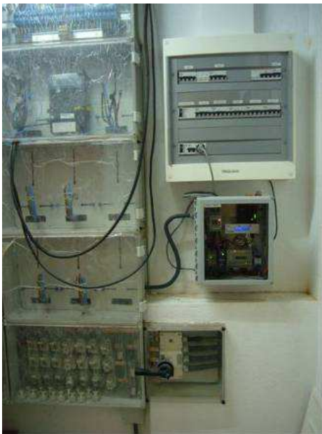
Figure 2 OPTIGES local controller installation in Barcelona
