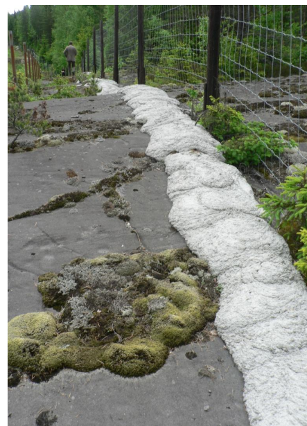
Figure 1. Cable shelter structure on the rock surface.
