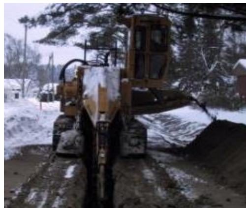
Figure 2. Trencher excavates frozen soil fast, but it cannot cut Finnish granite rock surface.
