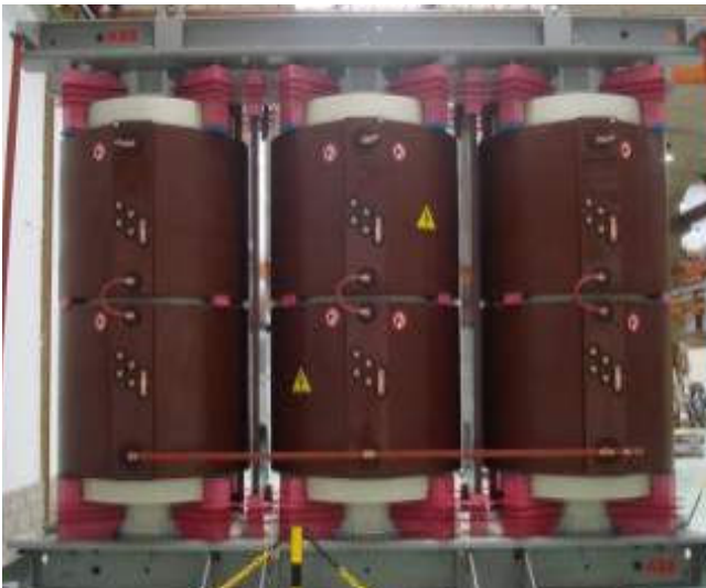
Fig. 1. New 66 kV/10 MVA dry-type transformer
