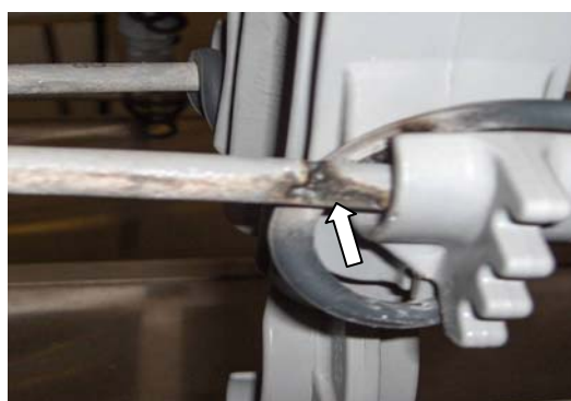
Figure 1 – Details of the typical kind of damage observed in a covered cable.
