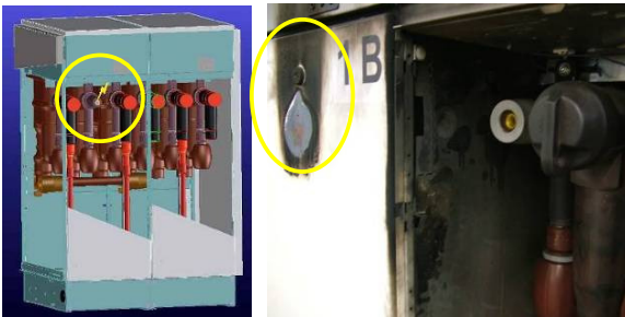
Figure 3 1-pole IAC test SVS, result after 2,65 kA-1s
