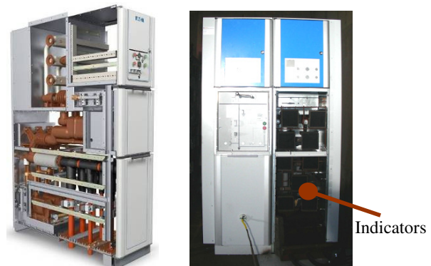
Figure 4 FMX, indicators in opened cable compartment
