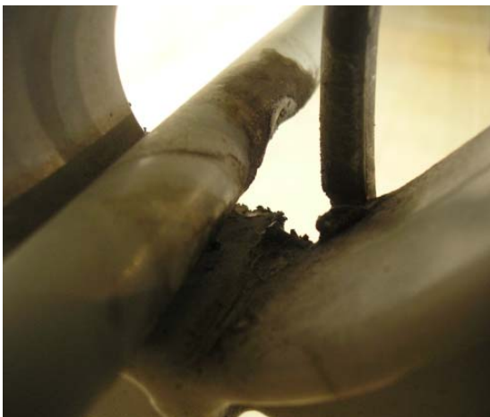
Figure 2 – Erosion for cable, spacer and fixing ring
