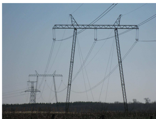
Figure 1. overhead power line
