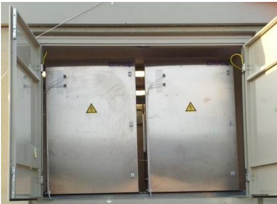
Figure 3. Two inverter cubicles as seen through a side door of the SSU.
