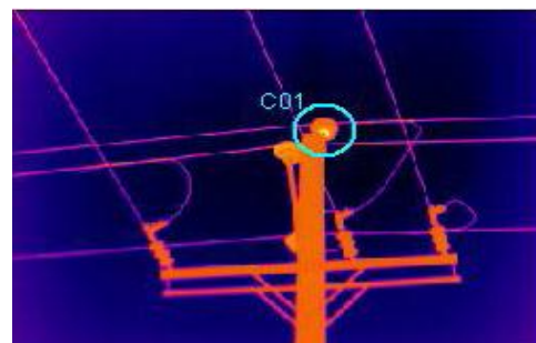
Figure3. An example of IR defect detection of in-service insulators In field inspection step long time leakage current
