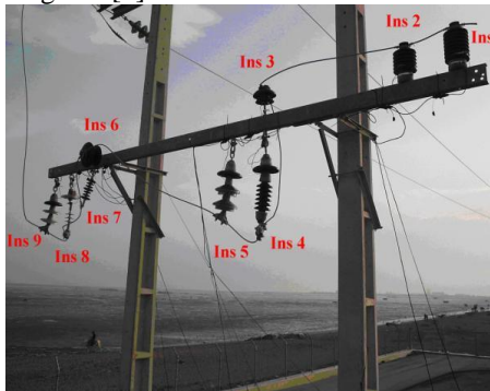
Figure 4. Online leakage current monitoring
