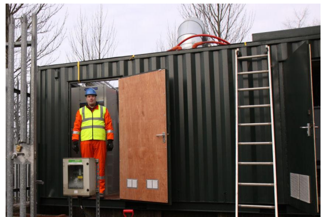
Figure 2 Pilot 2 SFCL during installation
