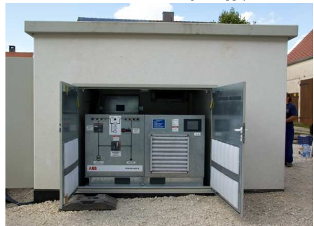
Figure 5: The "Smart Module", view towards the AVR
