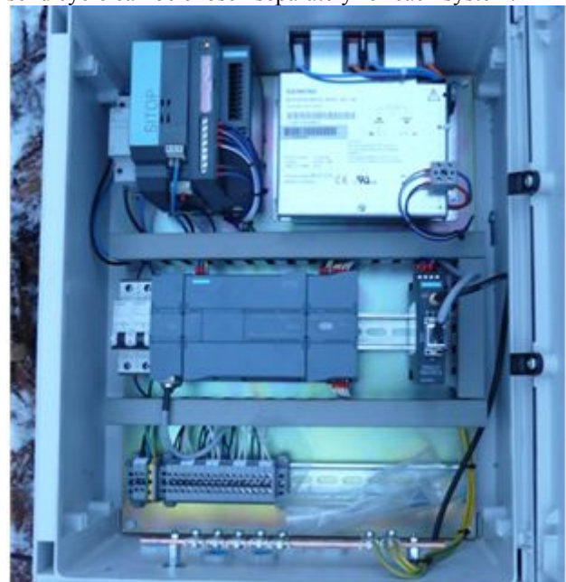
Figure 1: on-line PD monitoring system
