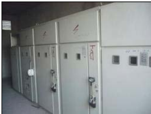
Figure.8: Proper anchor of switchgear in Ground substation
