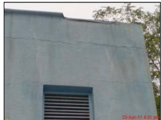
Figure.10: Cracks in substation Building Walls
