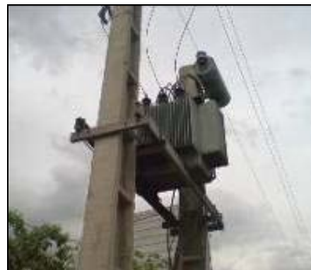
Figure.5: lack of anchor in overhead transformer
