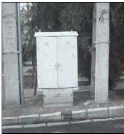
Figure.7: Proper anchor of switchgear to foundation in overhead substation
