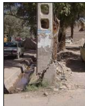
Figure.1: Shear failure in distribution pole (Bam, 2003)
