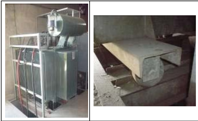
Figure.6: lack of anchor in ground transformer's wheel
