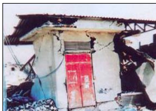
Figure.2: Collapse of substation building (Manjil, 1990)
