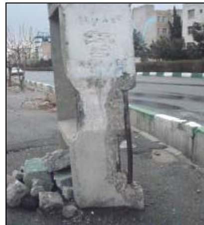
Figure.11: Concrete crush in overhead distribution pole
