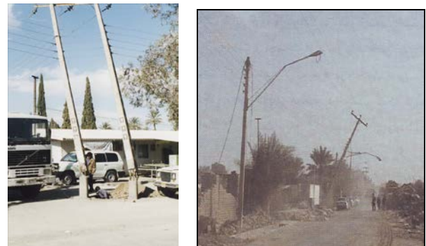
Figure.1: Bending failure (left) and significant rotation in soft soils (right) in distribution pole (Bam, 2003)
