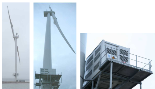
Figure 5: Example of a substation at the base of a wind turbine mast.
