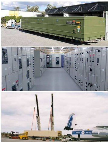
Figure 8: Complex installations in prefabricated enclosures (28 m * 7 m) tested prior to delivery.
