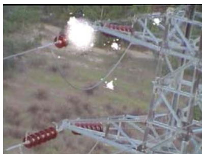
Figure 6 – UV inspections - damaged ceramic insulator
