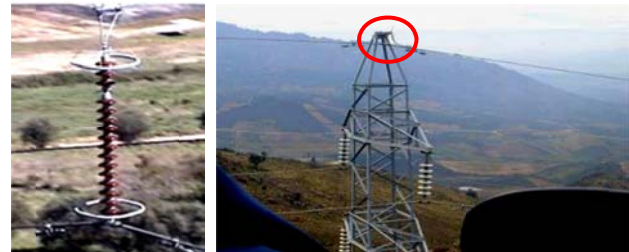
Figure 4 – Broken insulator; broken ground wire
