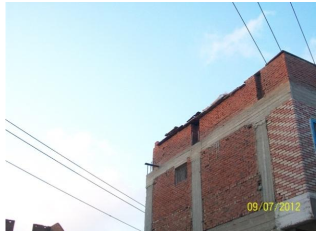
Figure 8. The Overhead power line location in Case study III
