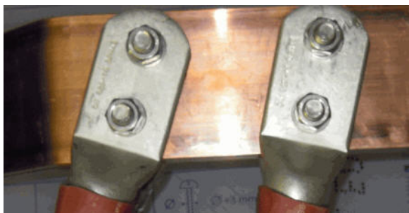
Figure 2: Example of tin-coated cable shoes connected to a bare copper bar
