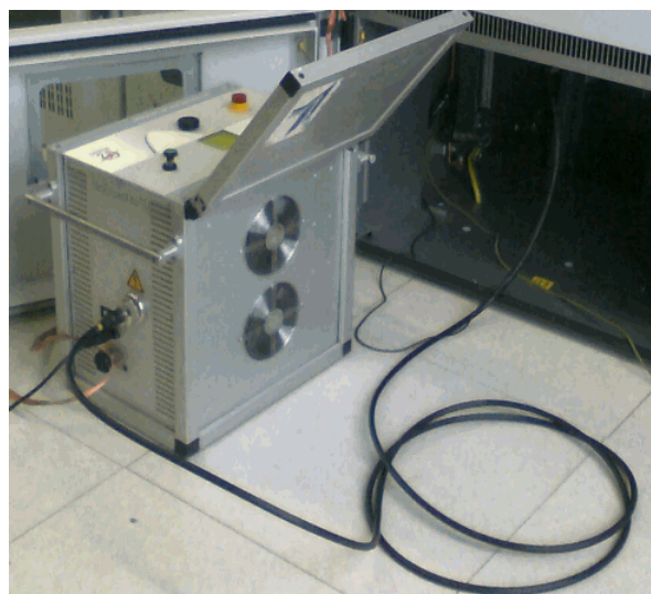
Figure 3: on-site 0.1 Hz cable test on newly installed MV cables, connected to the switchgear
