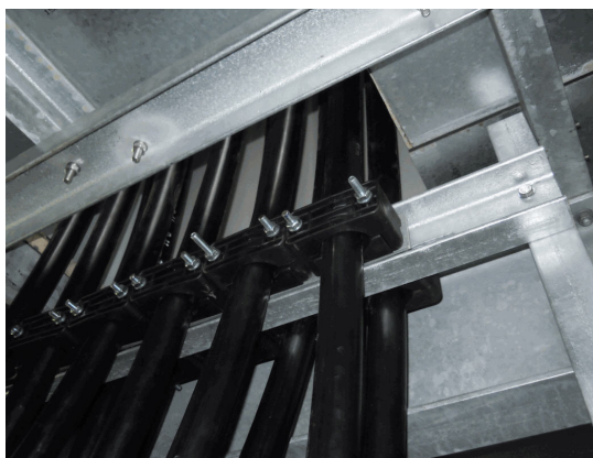
Figure 1: Cable fixations under switchgear cubicles
