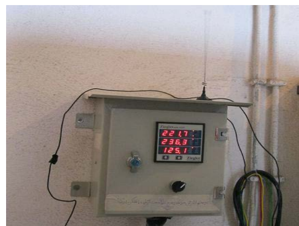
Fig. 2: a prototype of the device designed for the purpose of transformer status monitoring and operation of breakers in case of emergency conditions
