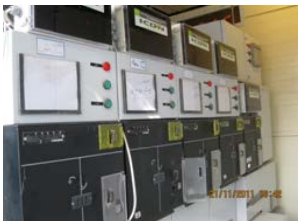
Fig. 3: An image of the equipments installed on MV
