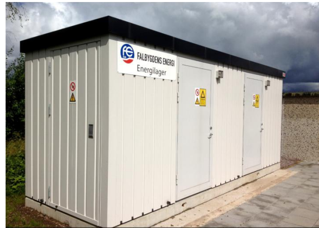
Figure 1. The 75-kWh battery storage in Falköping.
