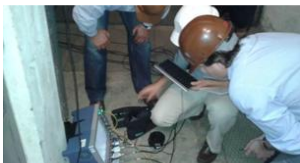
Fig. HVPD-Longshot™ unit in use by EDP engineers
