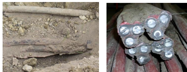
Figure 1: Melted cables and dry soil around
