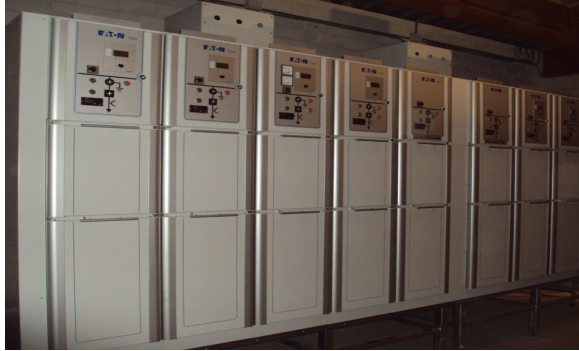
Figure 4 Switchgear type Eaton PowerXpert FMX integrated in Hitec Power Protection Data Center solution at Achmea Campus, Apeldoorn, the Netherlands
