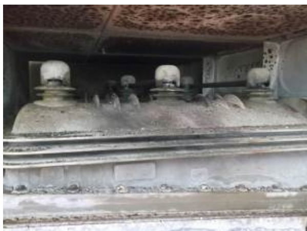
Fig. 3 – Example of severe degradation
