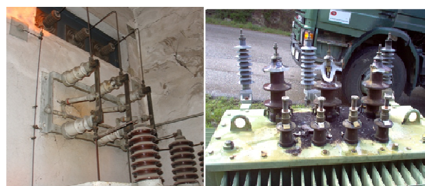
Fig. 2 – MV/LV Substations Typical Failure Mode
