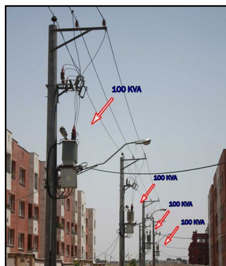
Figure 10. Use less power transformers 100KVA instead of using a high-power transformers such as 400KVA
