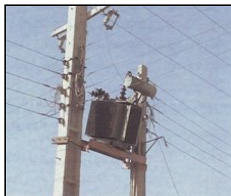
Figure 1. The transformers are falling and the bushings are breaking
