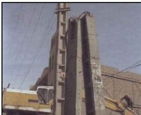
Figure 4. The breaking of electricity poles Particularly in the lower and
