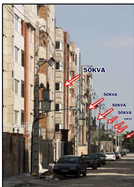
Figure 11. Use less power transformers 50KVA
