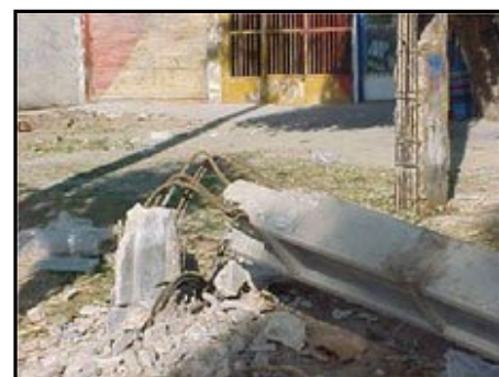
Figure 3. Square concrete pole break down in Bam earthquake
