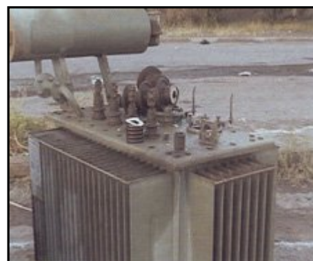
Figure 2. The falling of transformers from the pole and the breaking of bushings
