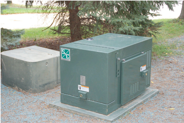
Figure 1: This 25-kVA Community Energy Storage unit is part of a large-scale installation serving many homes.
