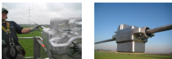
Fig 3: Installation of the smart grids sensor Ampacimon on a 150 kV line in the north of Belgium, near the North Sea.
