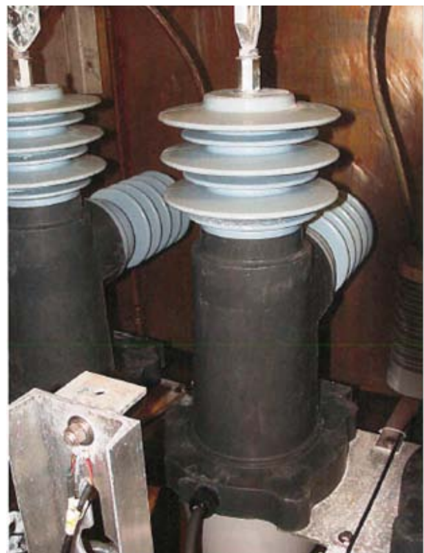
Figure 5: 1000 Hour Multi-Stress Test Lastly one switchgear unit is currently undergoing a 1
