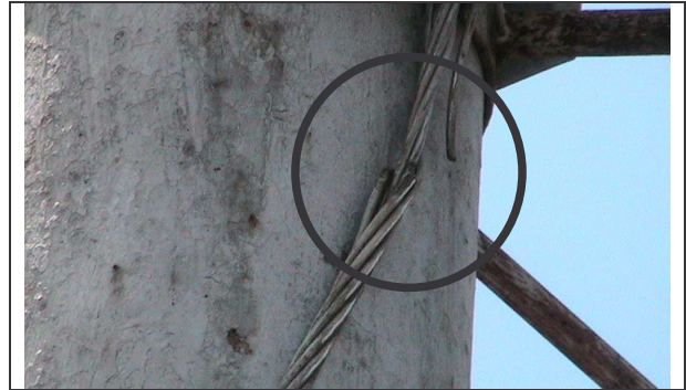
Photo 2: Snapped Strands of Steel Down Lead Conductor
