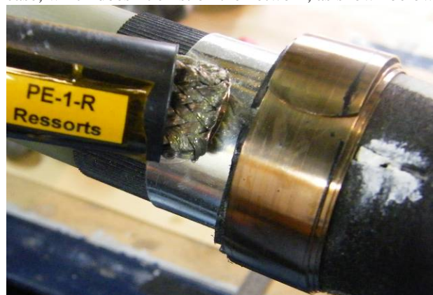
Fig. 4: Roll spring installed instead of collar-tie
