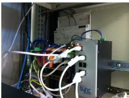
Figure 4 – Equipment installed for the demonstration project
