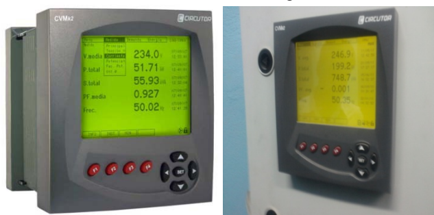
Fig 2: The CVM installed in the paint substation transformer
