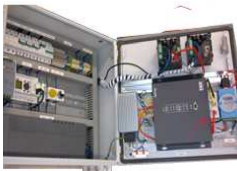
Figure 5: Cabinet with all system equipment
