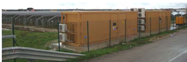
Figure 2. Picture of the inverter and storage containers
