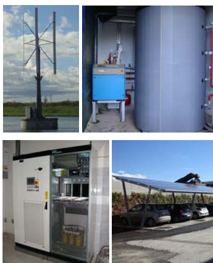
Figure 5. Wind turbine, cogenerator and thermal storage, electric storage inverter and PV plant
