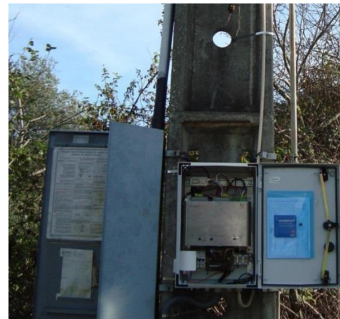
Figure 1 - Example of DTC installed in Pole MVS
