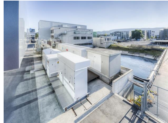
Figure 1: Top view of the Zurich 1 MW BESS.
