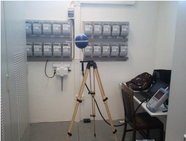
Figure 8 – Measuring EMF near smart meters.
