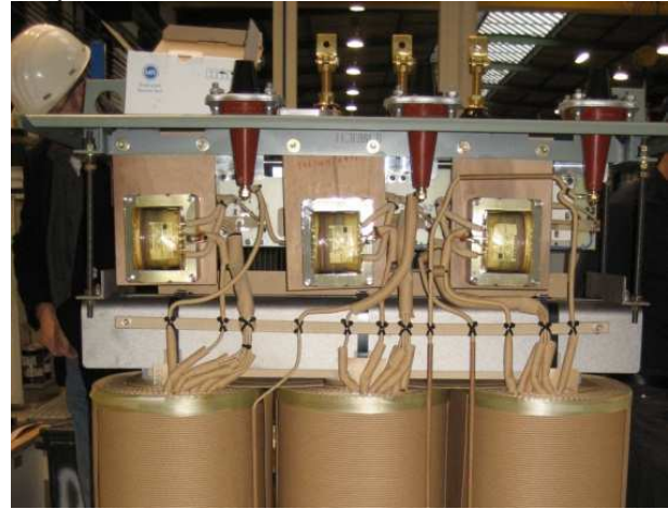
Figure 4 Reactor coils inside the Smart DT.
