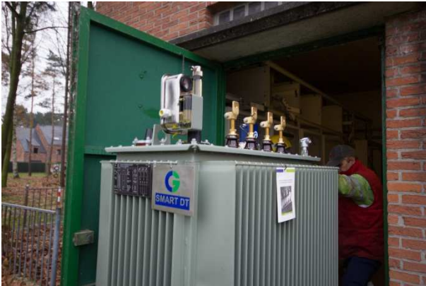
Figure 5 Installation of Smart DT in Belgium.
