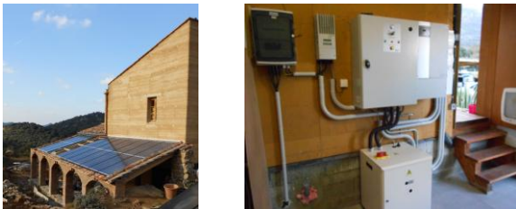
Photovoltaic panels (left), inverter and battery (right) of a Millener participant in Corsica
