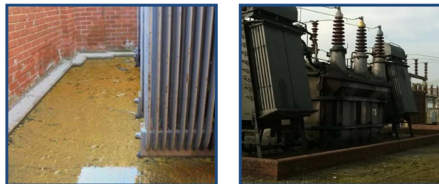
Image 3 – Bund containing oil spillage from primary transformer and grid transformer bund
