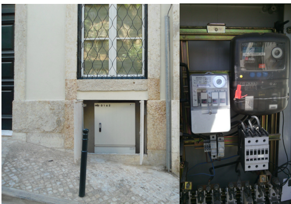
Picture 3 – Public lighting box with a smart meter.
