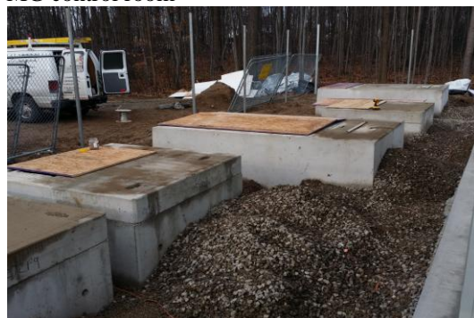
(b) Pad for container and incoming panel
