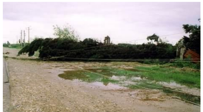
Figure 2: Falling of trees on medium voltage network in storm of oct.2015
