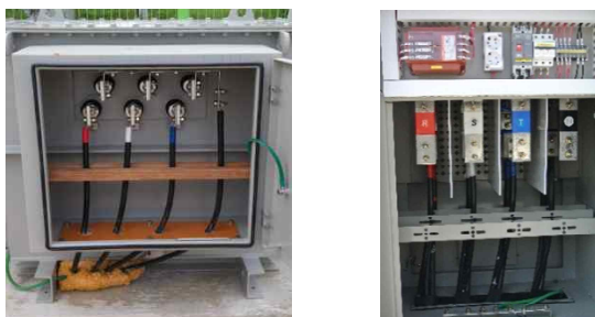
Figure 10. the fixed load and low voltage terminal unit
