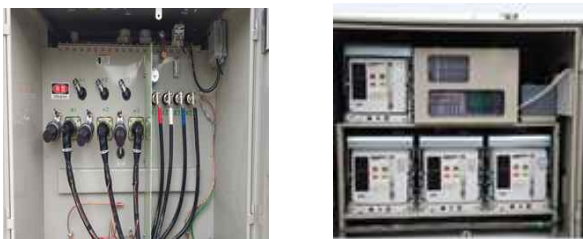
Figure 9. Transformer and ACBs with IED
