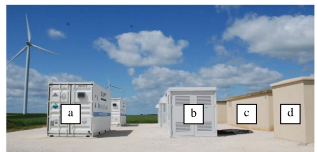
Figure 1: the DESS designed, built and operated within the framework of VENITEEA.
