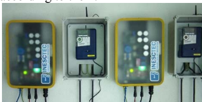
Figure 4 – Smart solar inverter prototypes and smart-meters installed
