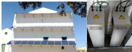
Figure 2 – PV panels and 2 of the 8 battery packs installed
